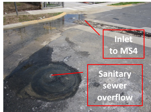
Wastewater flowing from a sanitary sewer access manhole to a nearby storm drain system inlet. Photo: PG Environmental
